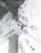
conduits running through Column Line B
